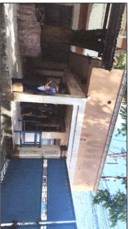
EXISTING GUARD HOUSE NOTE: FOR REPAINTING OF WALLS AND REPAIR OF CEILING
