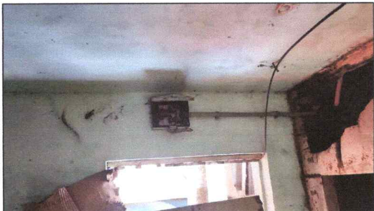
EXISTING ELECTRIC FUSE BOX NOTE: REPLACE WITH PANEL BOARD W/ BREAKERS
