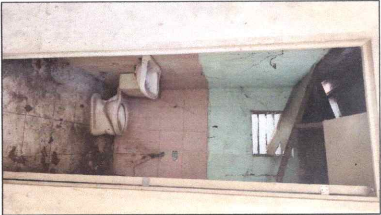
EXISTING COMFORT ROOM NOTE: RETILING ONLY ON FLOORS AND INSTALLATION OF NEW FIXTURES
